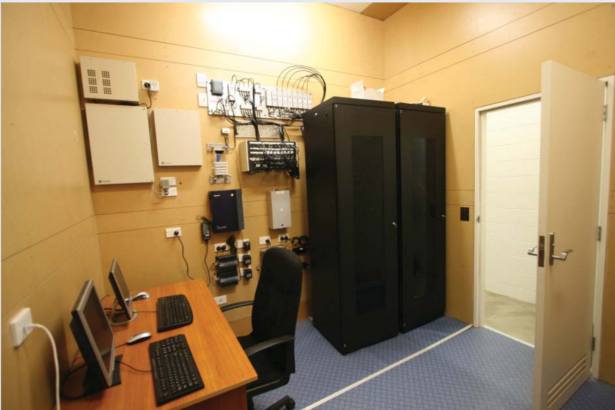
The Central Distribution Point.
